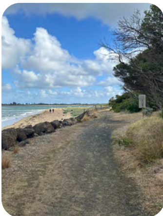
The foreshore trail is an important link in connectivity to both regional walking trails and local destinations, but is poorly kept and not DDA compliant.
