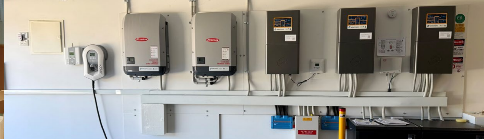
Additional solar PV 25.5 kw and a 2nd EV charging station installed in Werner's home
